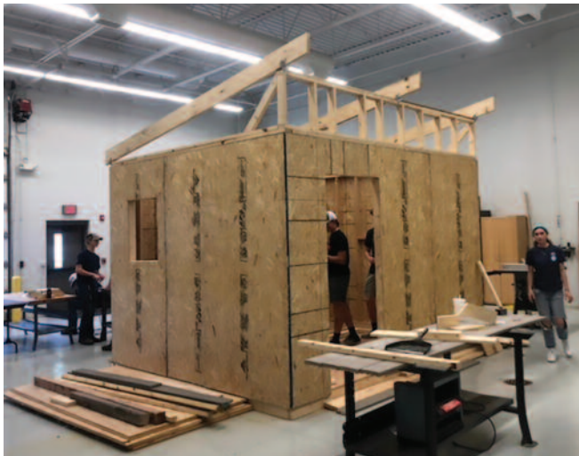
The $300,000 Illinois WorkNet grant is providing free apprenticeship training in building trades for nearly 30 students at DACC this year. Plumbing and carpentry will be two of the featured certifications in the program. Shown here are DACC College Express students building a miniature house.
